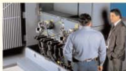
COOPER Power Systems
